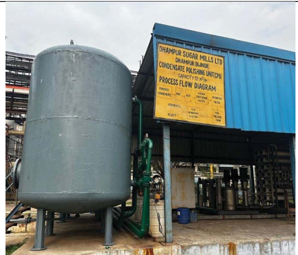
Fig 8: Condensate Polishing Unit
