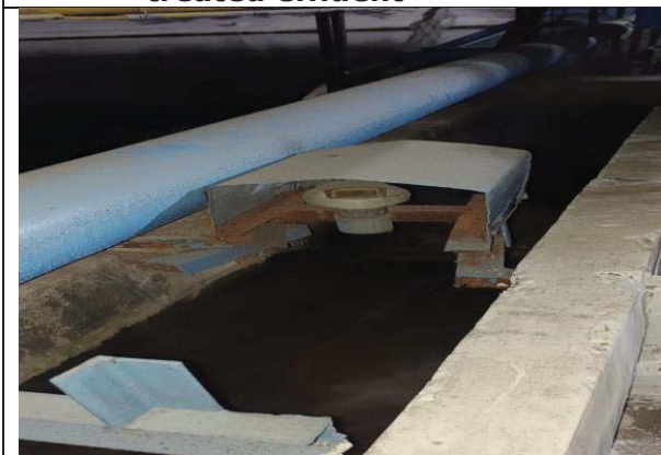
Pic: 5 Flow meter at the inlet of ETP
