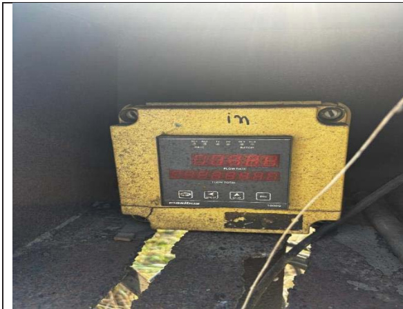
Pic 1: Flow meter at the inlet of ETP
