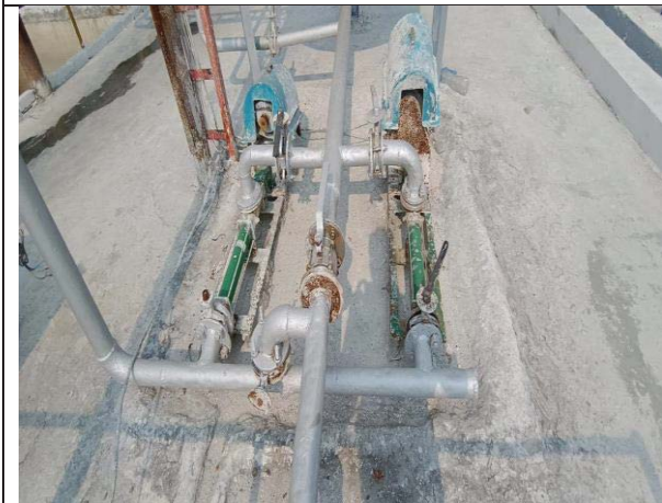
Pic: 7 lime dosing pump
