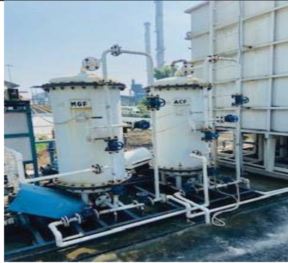
Pic: 11 MGF and ACF units of STP
