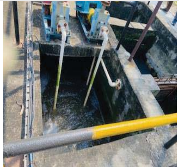
Pic: 10 STP inlet
