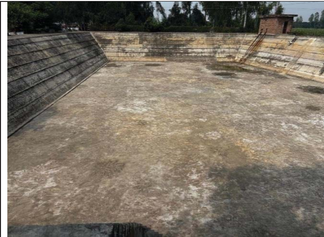
Fig 1: 10000 m3 brick-lined lagoon
