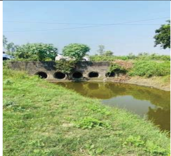
Pic 16 : Rain water accumulated in River SOT
