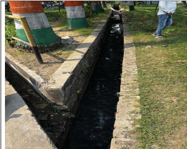
Fig 7: City drain for seage within unit premises
