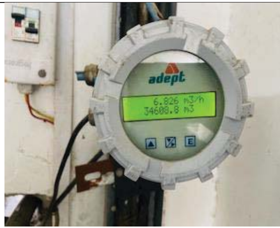
Pic: 8 Flow meter at the inlet of STP
