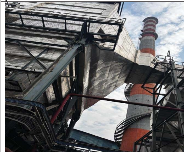
Fig 9: Common stack for both boilers
